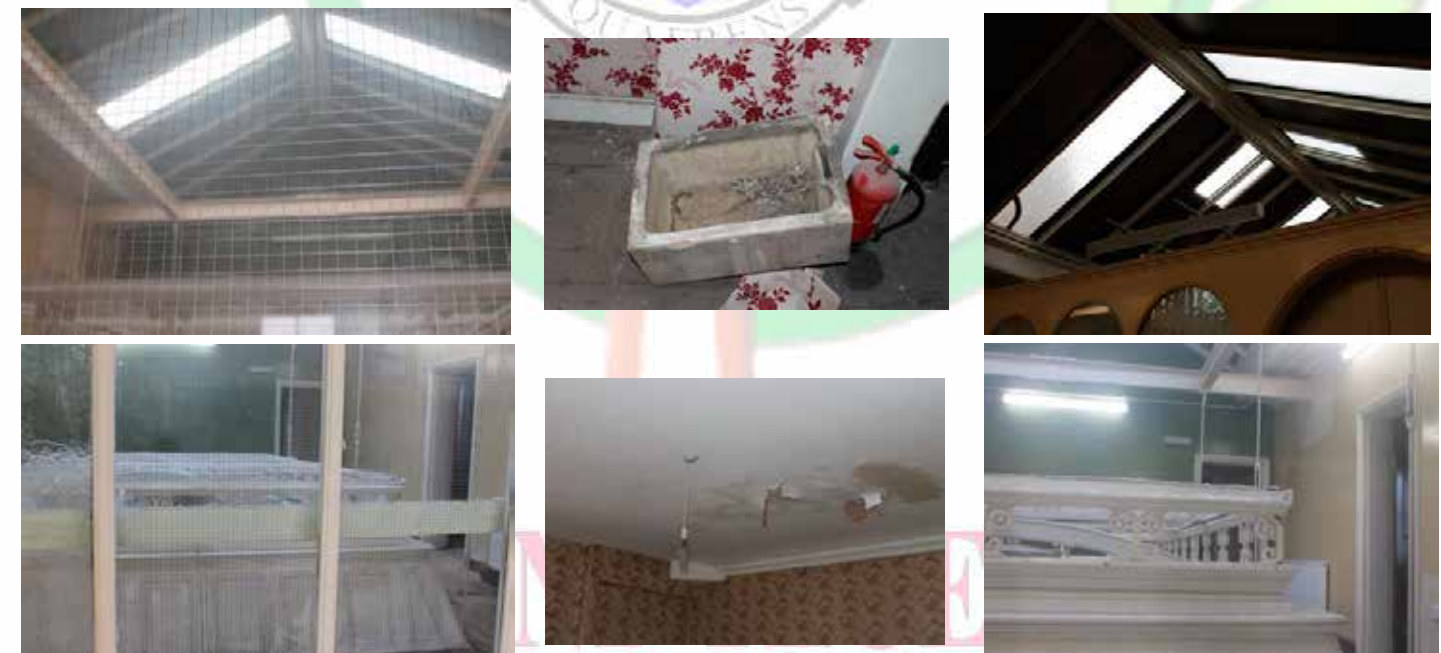
Existing conditions of the upper floor where extensive refurbishment is required. A covered external fire escape and vertical access lift would also need to be installed
