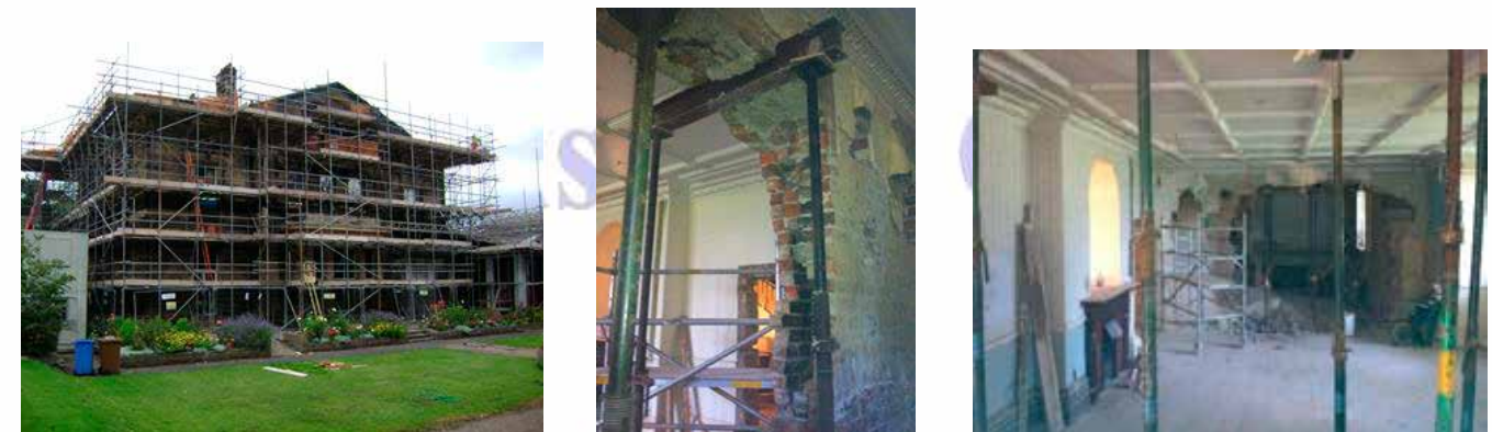
Some of the refurbishment works which were carried out under Phase One
